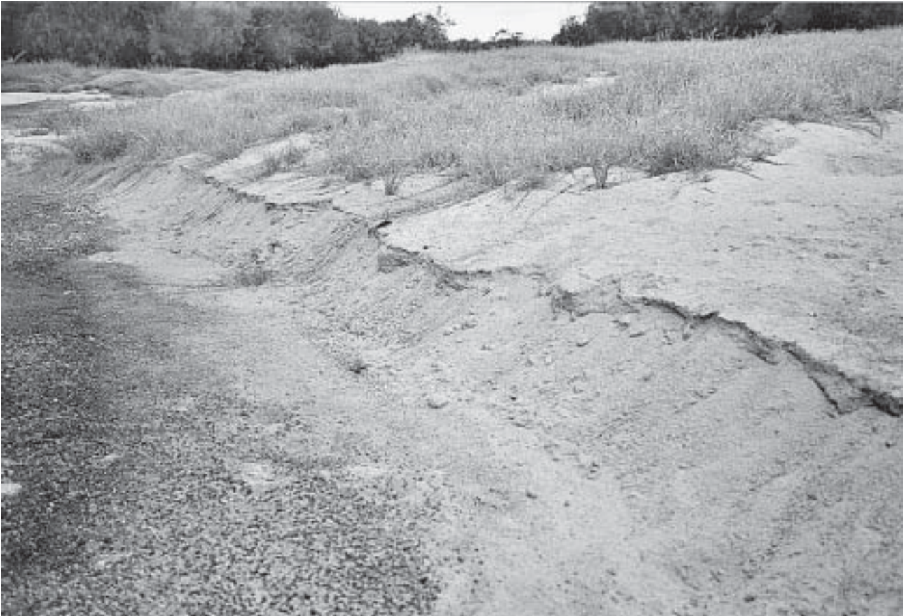
Photo 10. Unconsolidated sediment upstream of the pool.
