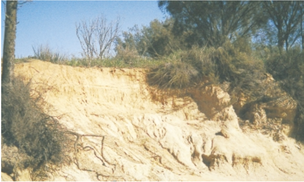
Severe bank erosion occurs in some sections where the channel is more defined.
