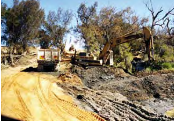
Sediment being removed from Railway Pool and transported off site (Photo courtesy Nina King)
