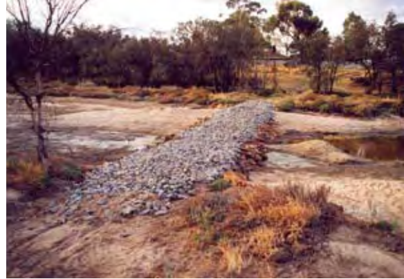
Riffle constructed upstream of Beverley Town Pool to trap sediment (Photo courtesy Bernard Kelly)
