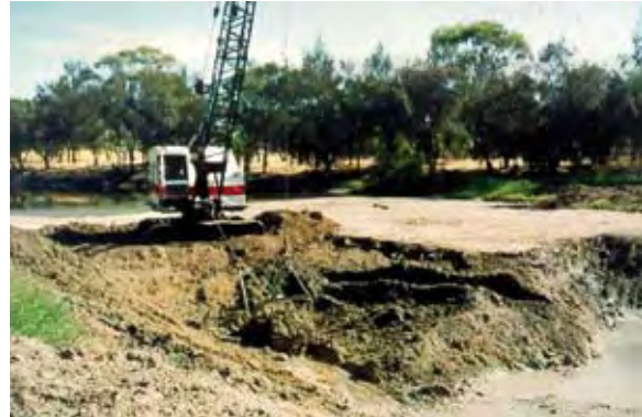
A dragline removing sediment from Beverley Town Pool in 1993 (Photo courtesy Fred Bremner)
