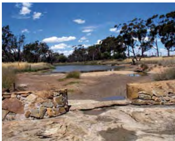
Weir-like structure at the downstream end of One Mile Pool. (Photo courtesy Prue Dufty)
