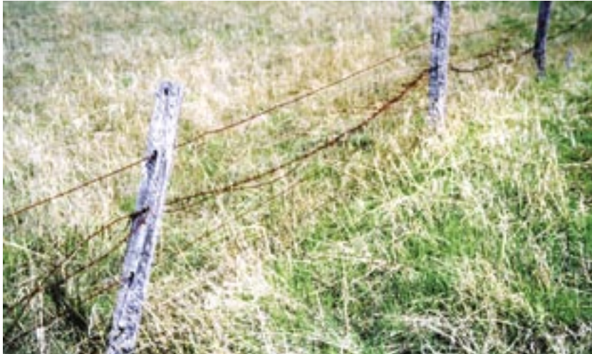
Fence in poor condition
