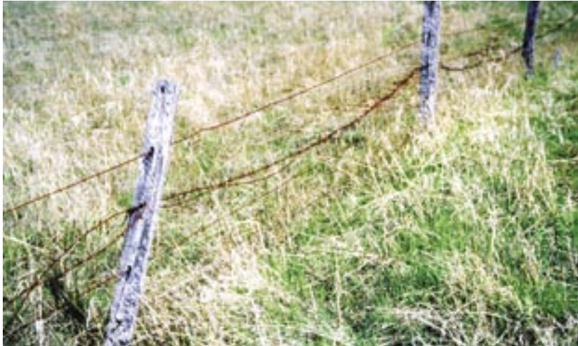
Fence in poor condition
