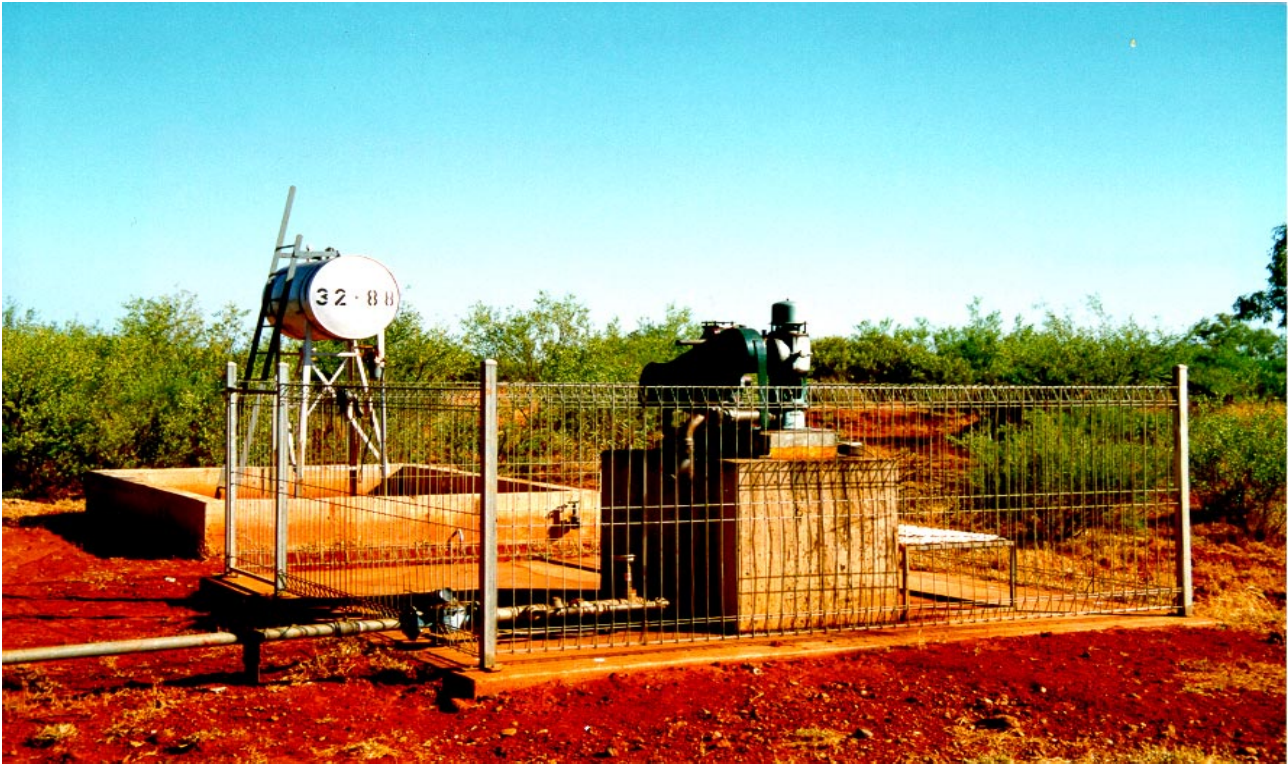
Plate 1. Diesel fuel storage at bore 32/88
