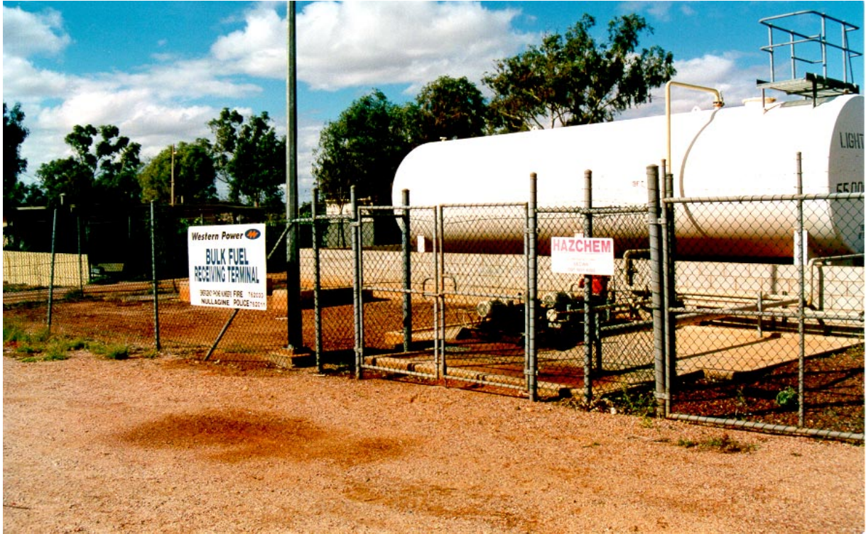
Plate 3. Diesel fuel storage at the Western Power Station
