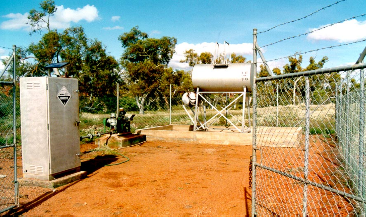
Plate 2. Diesel fuel storage at bore 1/91
