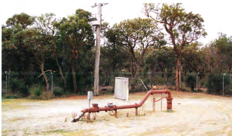
Water supply production bore in Jandakot, Western Australia Photographer: Mr A Tomlinson
