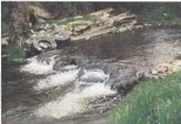
Plate 13. Bed/riffle control structure across the Great Forester River, Tasmania, made by the Springfield Landcare Group from truck tyres wired to pig netting fence.
