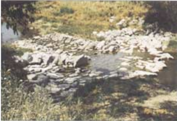
Plate 12. The Cockburn River near Tamworth, New South Wales, looking upstream from the right bank. A rock-bed control weir and fishway are being used to prevent bed lowering in a stream on which sand and gravel mining has been excessive.
