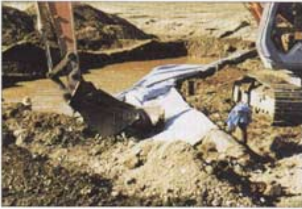
Plate 7. Constructing an experimental log sill in the Nambucca River. The geo-textile membrane reduces undersill seepage and raises the watertable level of the stream.
