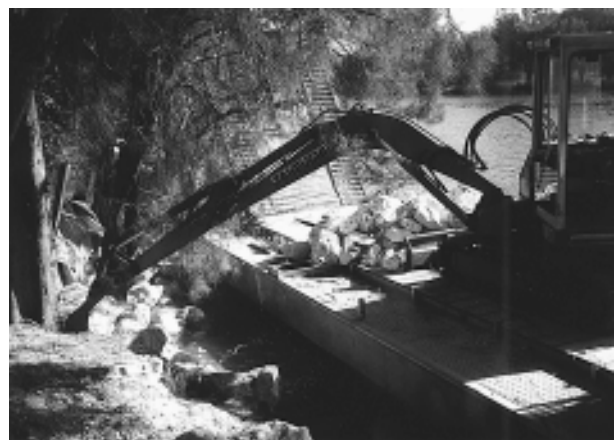
Erosion control works were undertaken by the Swan River Trust to protect river banks and trees along a 35 metre section of foreshore in Bassendean.
