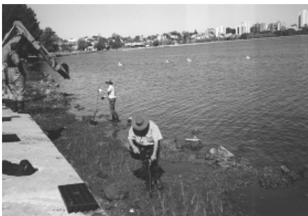
Swan River Trust crew at Sir James Mitchell Park, South Perth planting 1000 reeds.
