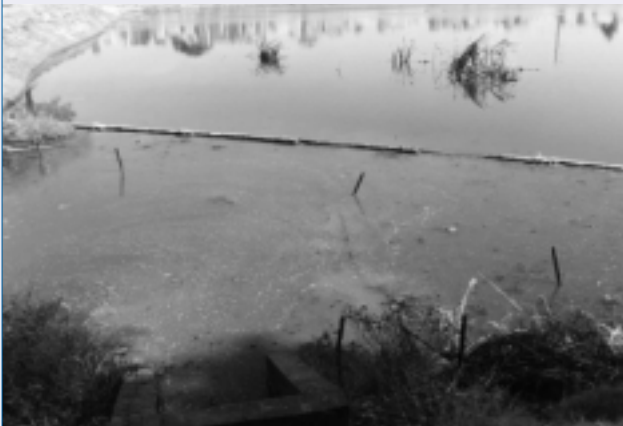
A poorly managed industrial stormwater drain entering a compensating basin in the Mills Street Main Drain network.
