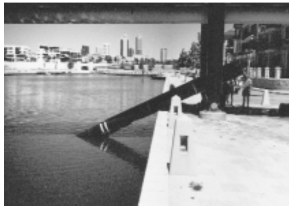
The Claisebrook wastewater pressure main, which was attached to the underside of the Claisebrook Cove pedestrian bridge, collapsed into the Claisebrook Inlet on 26 November 1999.
