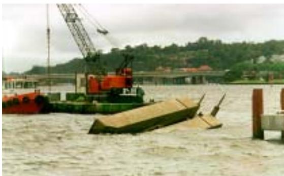
Overturned barge at Barrack Square in October 2000. The barge was performing dredging to accommodate the construction of a jetty as part of the Barrack Square redevelopment.
