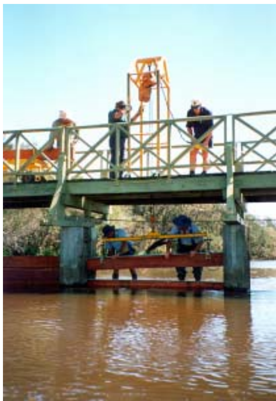
Trust field crew installing the Kent Street Weir boards in October to stop salt-water flowing upstream of Kent Street in the Canning.
