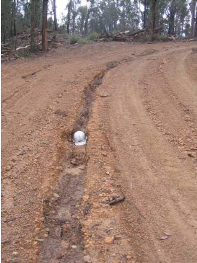
An example of major water related erosion
