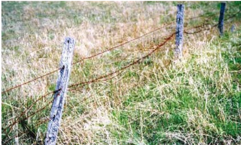
Fence condition: POOR.
