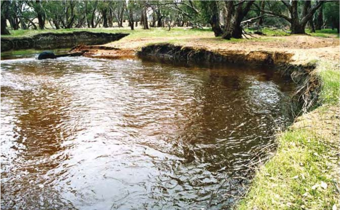
Image 10. Incorrect placement of this crossing has caused it to be washed out and the banks to erode
