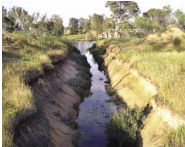
Photo 26: Drain confluence with Dwardadine Pool in Photo Section 16
