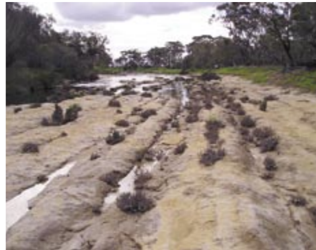
Photo 5: River bed scour resulting from River Training Scheme
