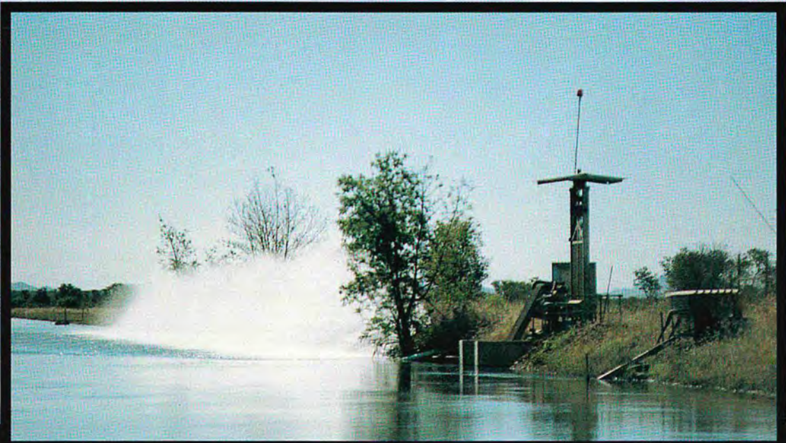
Photo 4: Cooling water from the Mill being returned to the M1 Channel
