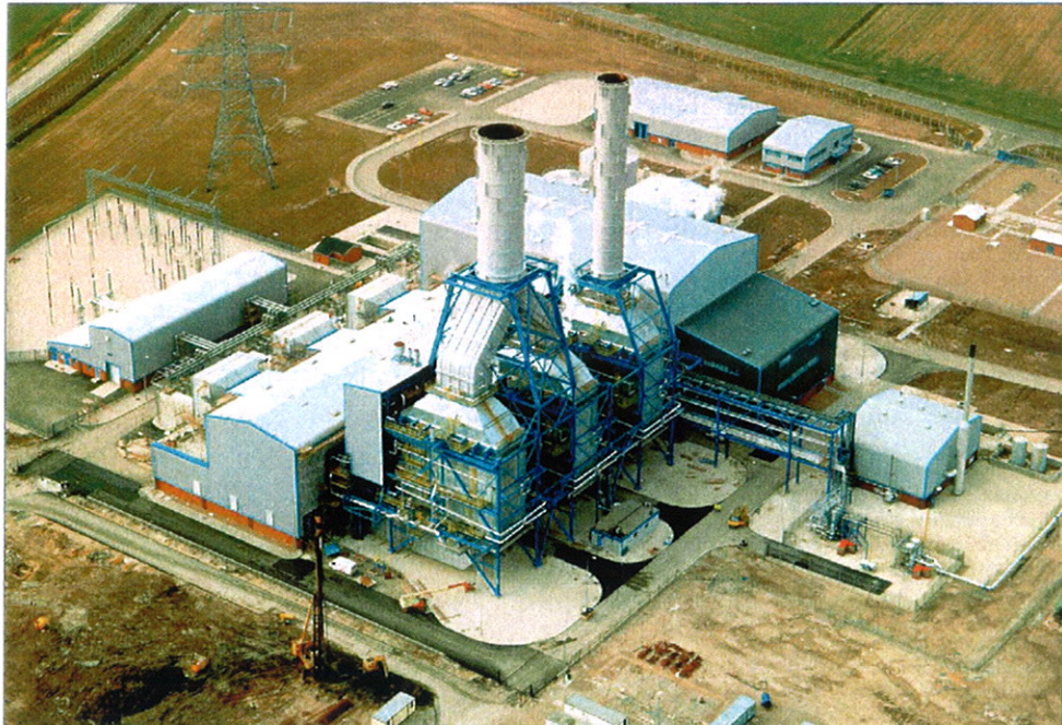
Construction of the first phase of South Humber Bank 750-MW combined cycle in England. Two HRSGs exhaust into one stack, foreground, the third boiler exhausts into a single stack. Unusual arrangement was required to meet local 'visual impact' environmental regulations.
